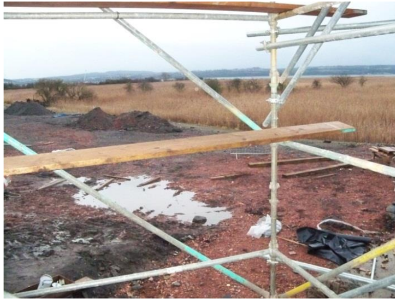
Figure 2 - Planks placed at the end of a scaffold
