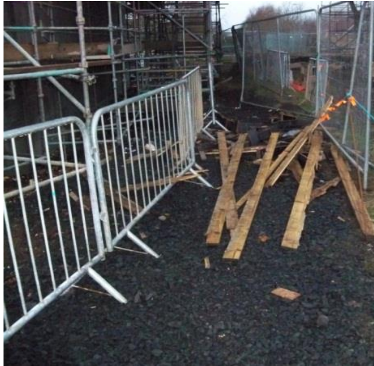
Figure 3 – Planks in the access route creating trip hazards
